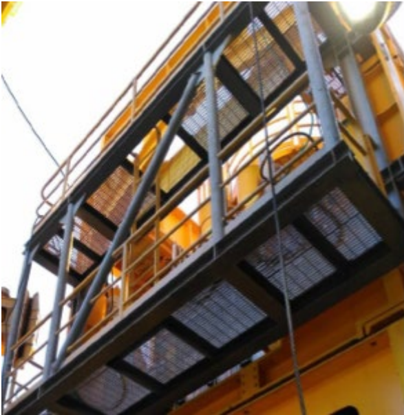
Area from which worker fell
